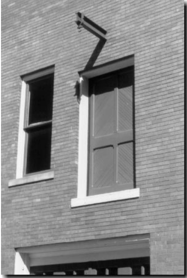
{ PHOTO 47 } This second floor door has been closed off with an appropriate door pattern for this building. Note the metal bar above the door; it was used to help hoist materials to the second floor.
