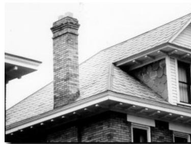
{ PHOTO 30 } Nicely preserved brick chimney. It has a corbeled top.
