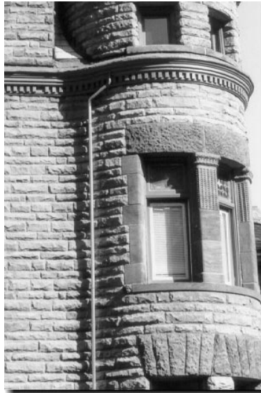
{ PHOTO 28 } This gutter is designed into the cornice detail and the downspout is tucked into a corner.
