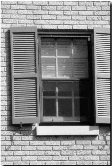
{ PHOTO 46 } Operable open shutters that fit the opening are held back by shutter dogs anchored into the brick wall's mortar joints.
