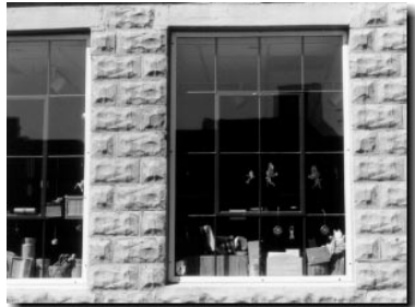
{ PHOTO 38 } Fixed commercial exterior storm makes the window inoperable. Note the thin metal frame around storm does not cover or obstruct the original window.
