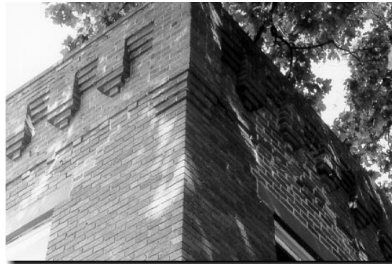
{PHOTO 14} A stepped or corbeled cornice. Note the recent repointing that does not match the existing mortar.
